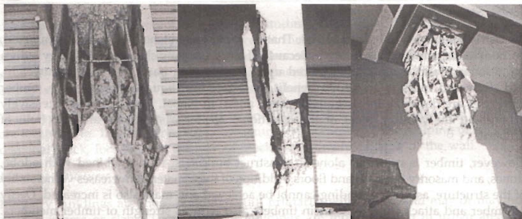
Photo 3. Details of damages in three front columns in Pooja flat in Anja, Gujarat.
