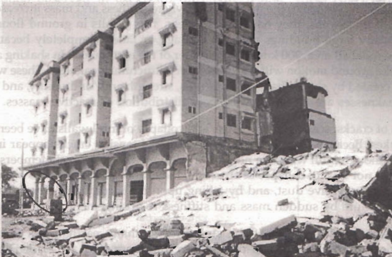
Photo 2. Pooja flat in Anja, Gujarat. Out of 4 wings, one wing collapsed completely and other three parts suffered structural damages. Details of structural damages in the marked area are shown in Photo 3.
