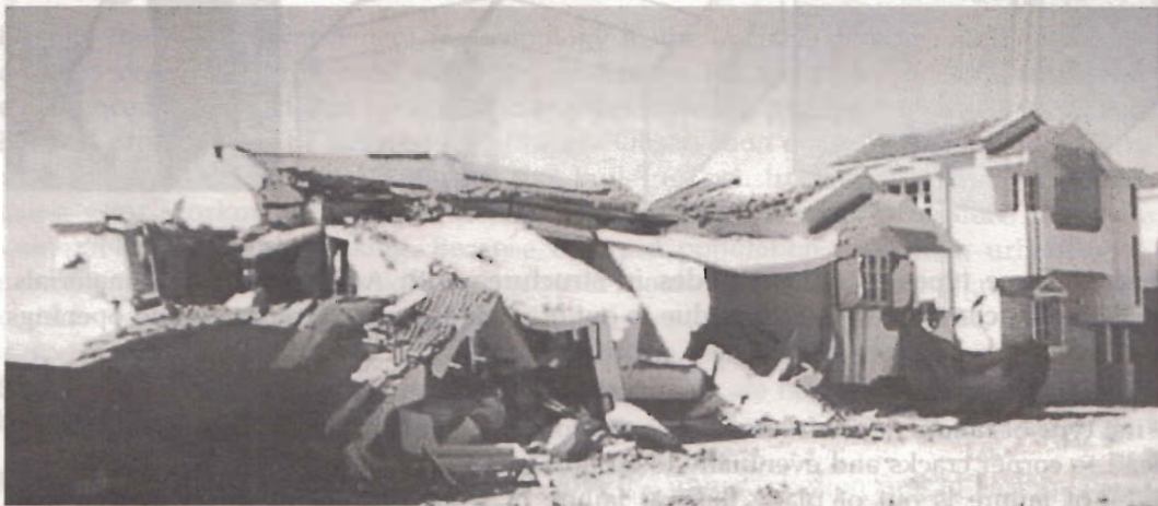
Photo 1. Failure of architecturally beautiful looking newly built residential complex from Gujarat earthquake.
